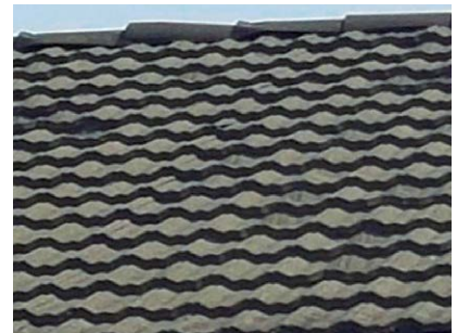
GERARD tiles after the hailstorm in Črnomelj*
