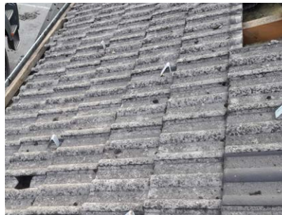
Concrete tiles after the hailstorm in Črnomelj*
