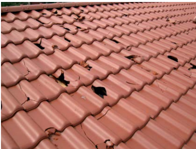
Clay tiles after the hailstorm
