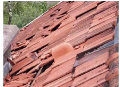
Clay tiles after the hailstorm in Črnomelj*
