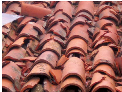
Clay tiles after the hailstorm
